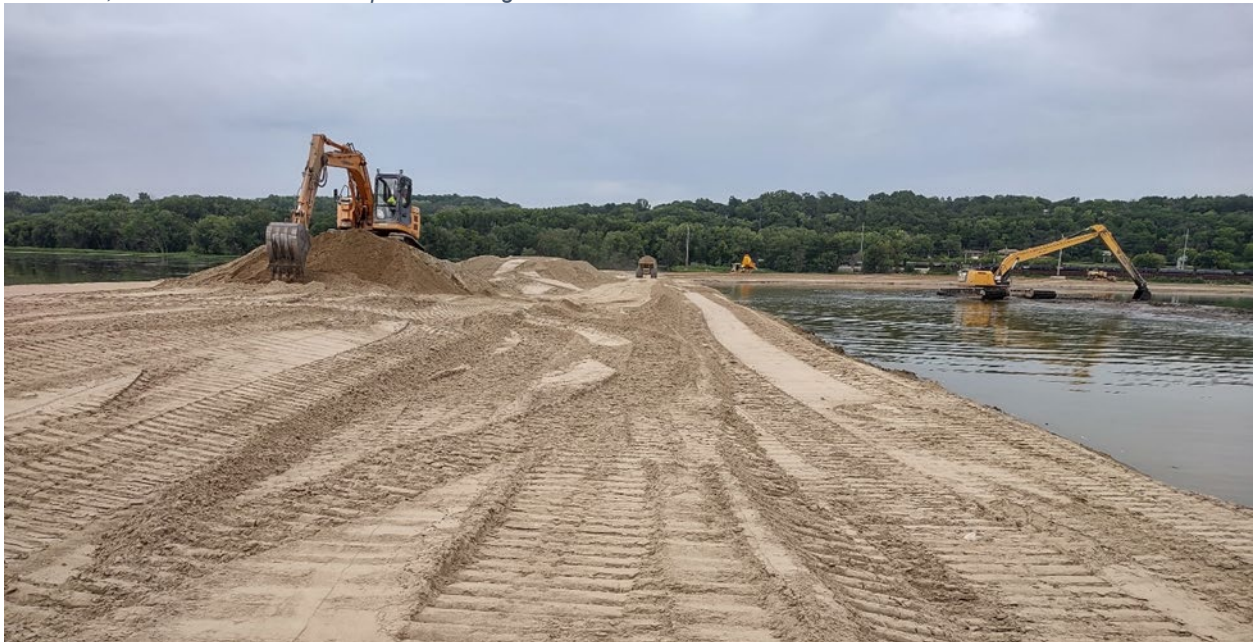
Figure 4: Earthmoving equipment is used to distribute granular material after settlement has occurred, to meet the final grade requirements. The long arm excavator on the right side of the photo is distributing sediment at the edge of the island; soft sediments were displaced during island construction.
