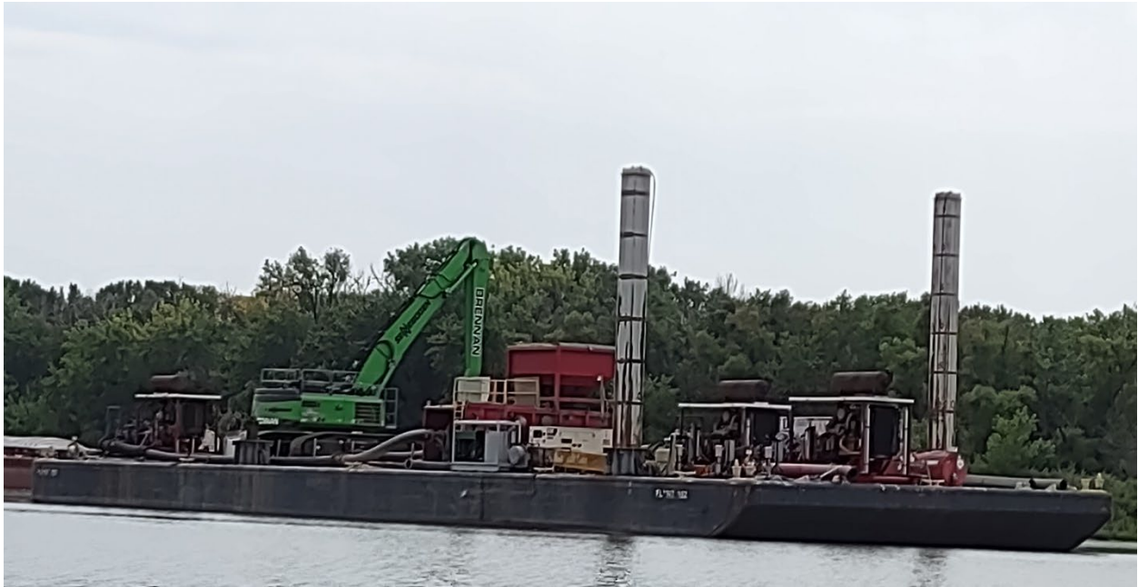
Figure 3: Brennan plant for placement. A shallow draft barge holds an excavator (green) for off-loading sediment from a barge into the red hopper. The sediment is pumped into place using hydraulic pumps.
